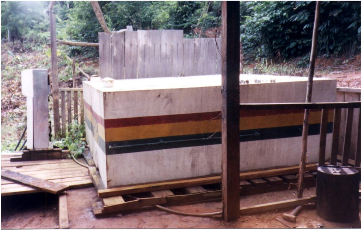
Figure 21: diesel oil container - 10,000l with electric pump
