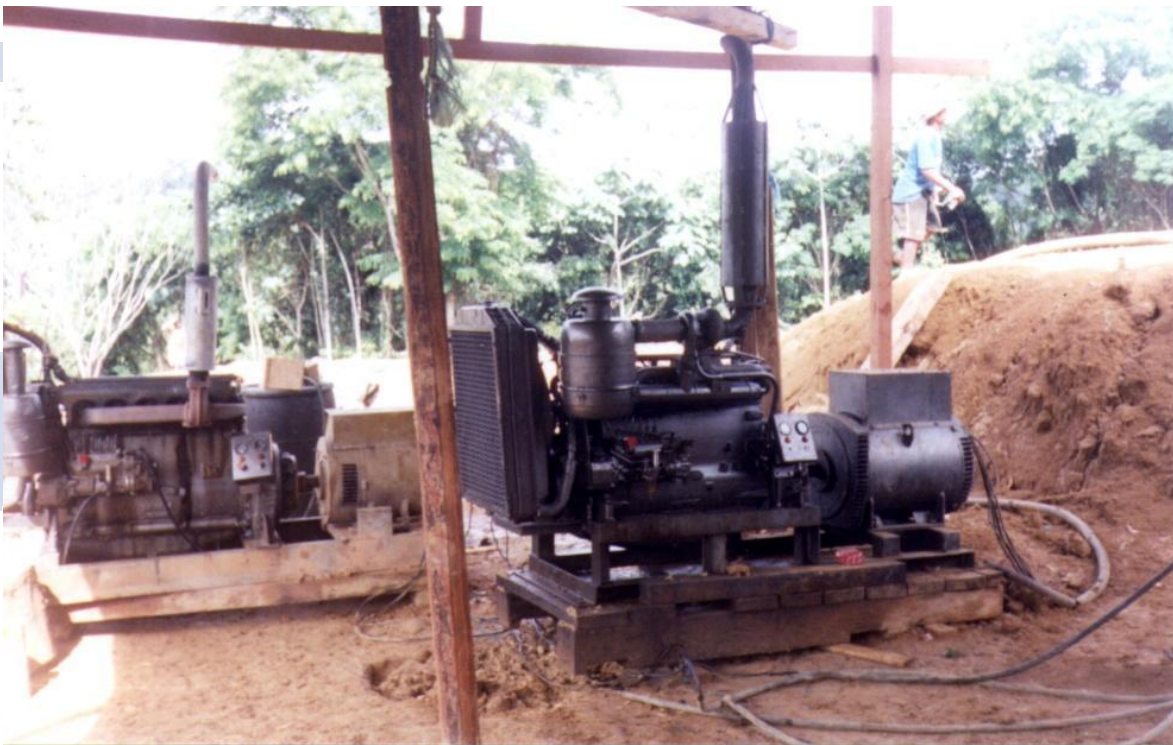
Figure 20: power generation units, motors 6c MWM coupled to generators 100 and 60 Kwa
